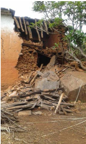
One of the damaged homes in Thulipokhari.
