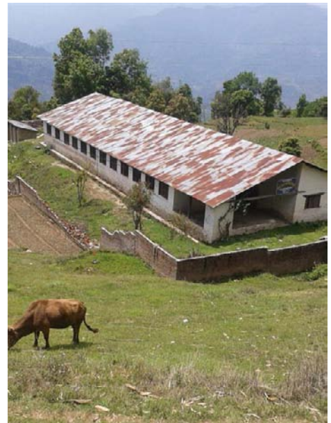
The Girls Dormitory in Thulipokhari suffered only minor damage. The security wall we recently had installed didn't fare as well in some spots.
