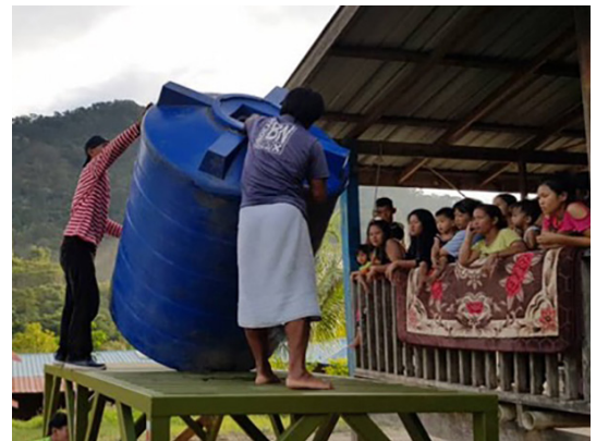
A large storage tank is readied for installation to harvest rainwater in rural Sarawak, Malaysia.
