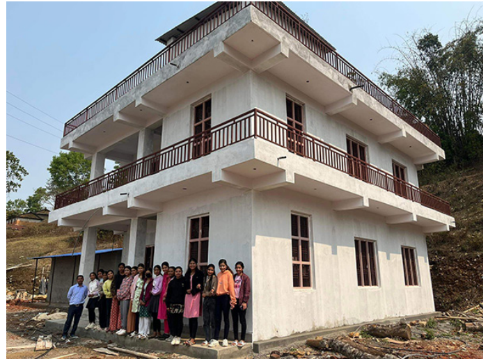
The new modern dorm has been constructed and needs furnishing for the girls in the fall.
