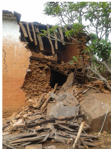
One of the many buildings devastated by the earthquake. The dormitory suffered cracks, but no major damage.
