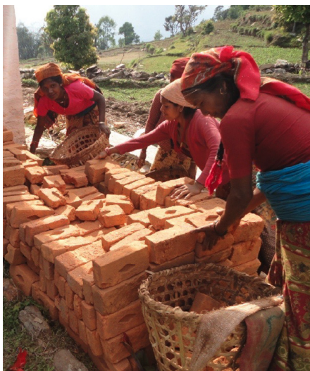
Once again, women from the village carried bricks for the wall construction.
